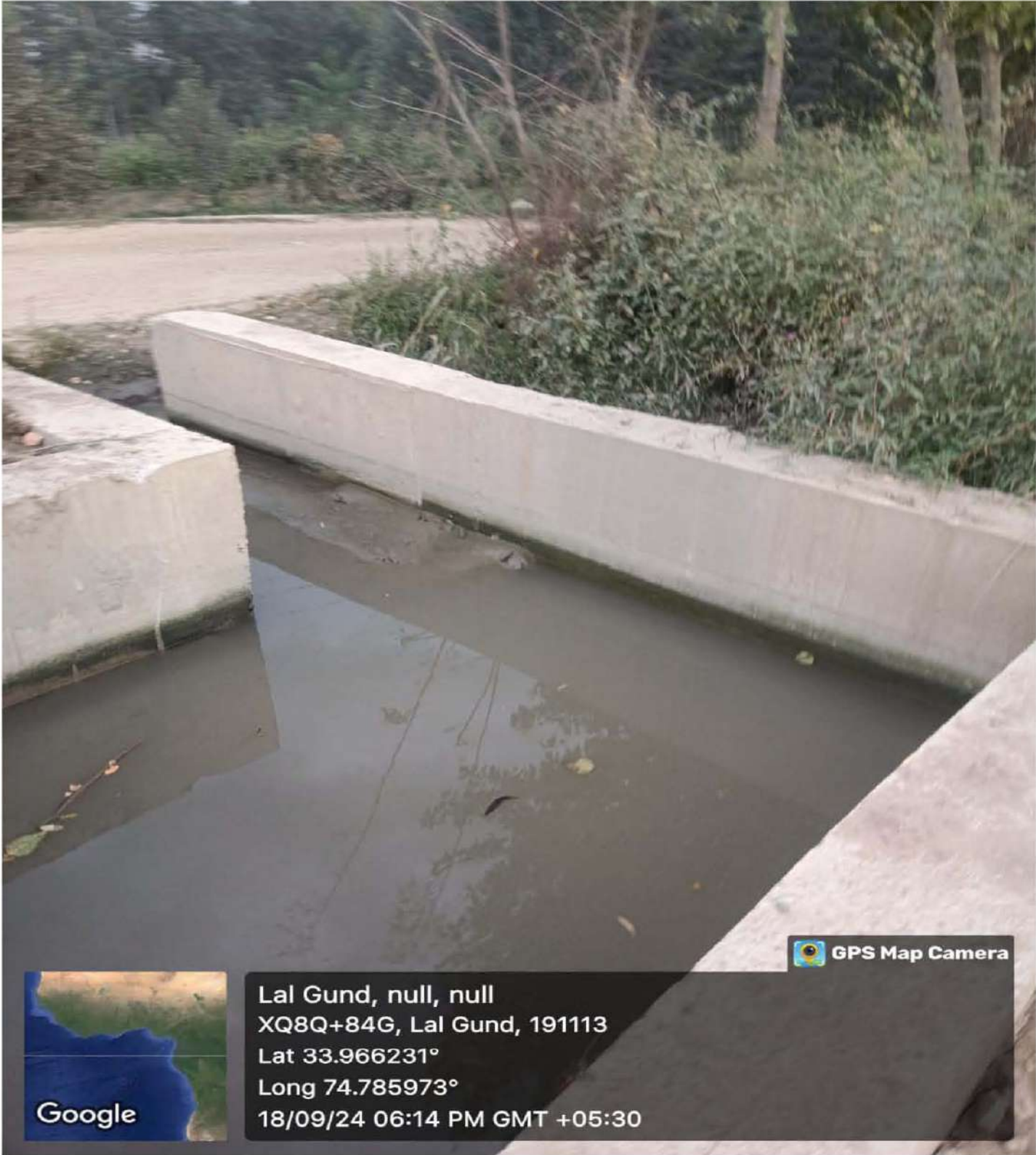
Water Channels at Atta Kul At Village Gudsthu Budgam Ch-16+300 Water flow free LHS To RHS by Syphon
